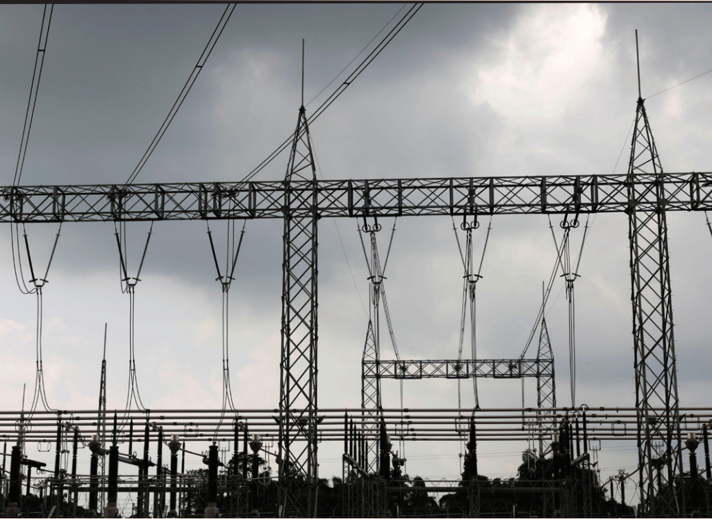
Electrical power lines at the natural gas-powered Azura-Edo Independent Power Plant in Benin City, Nigeria, June 2018. Nigeria has the capacity to produce upward of 12,000 megawatts of electricity each day but often dispatches only 4,000.
